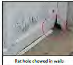
Rat hole chewed in walls
